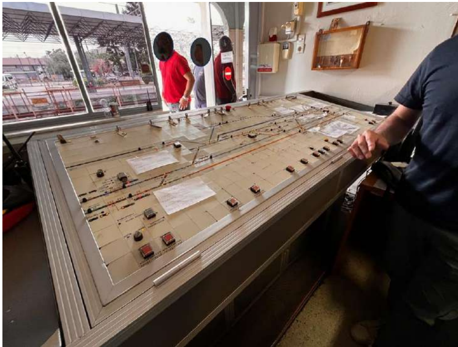
Figure 37. The control panel at Larissa Station
